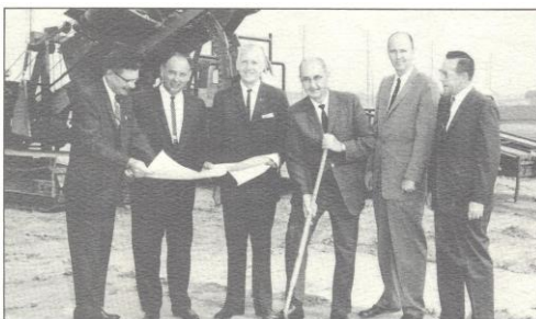
GROUND BREAKING - May 21, 1965. Commissioner Kenny Fagans is joined (from left) by Dr. Murrell Miller, Vern Furgerson, Executive Committee Chairman Robert D. Ashton, Gahr High Principal Willard Redfern and Charles Hutchinson, as ground is broken for the new CIF-SS Office in Cerritos. Miller, Furgerson and Hutchinson represent the Artesia-Bloomfield-Cerritos School District.
